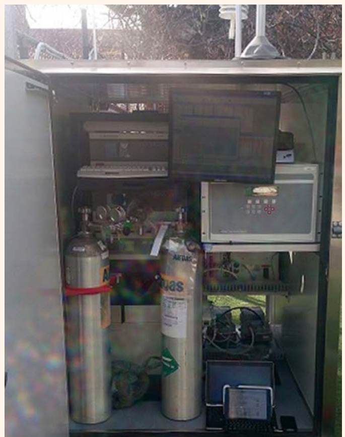
Figure 6: Clifton Hill Primary School - Air Quality Checking Station
